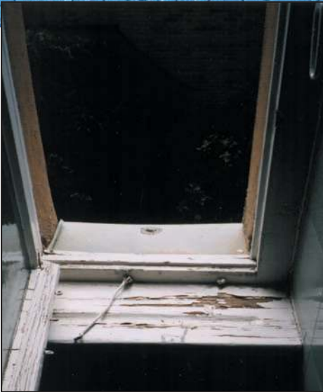
Leaky window – mold is beginning to rot the wooden frame and windowsill.
